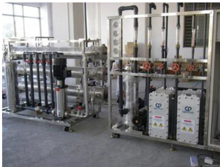
Water Purification System
